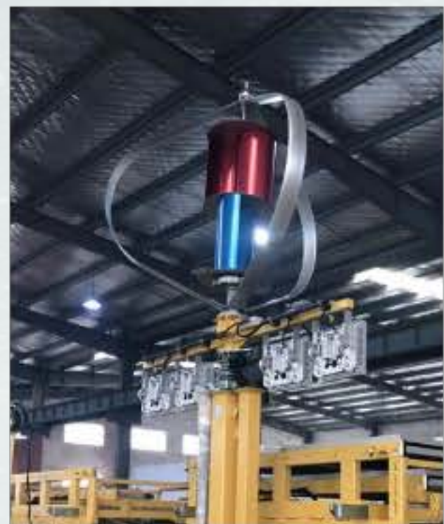
400W & 600W Wind Turbines
